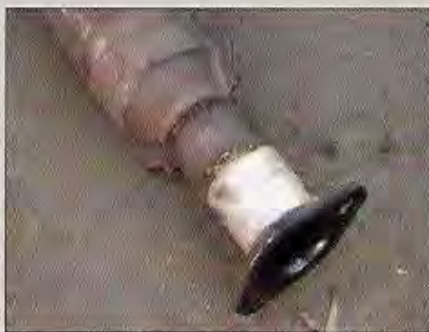
Notice how a different flange has been welded onto this pipe, plus it has extended a couple of inches.
